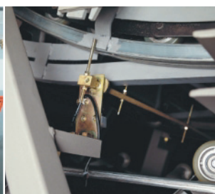
❸ Step Safety Switch
