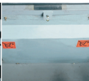
❷ Safety Guard at upper and lower machine rooms
