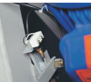
⑥ Driving Chain Safety Device
